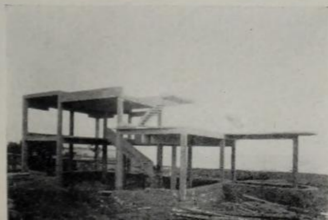
Fig. 129. Stamo Papadaki, 1932 Reinforced concrete framework for a two-story building (Athens, Greece) This skeleton can also be filled in with non-bearing opaque or with transparent glass walls. In spite of this, such frame structures are often handled as brick buildings, camouflaging new potentialities with obsolete schemes
