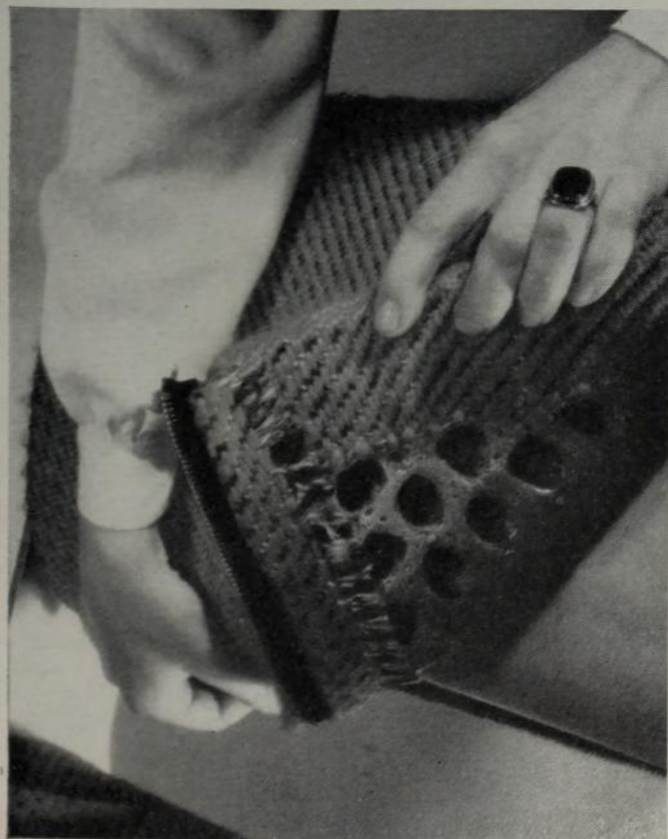
Fig. 92. The covering of the back with air foam, wrapped around the 1/8-inch plywood drum fastened between the two sides of 1/4-inch plywood
