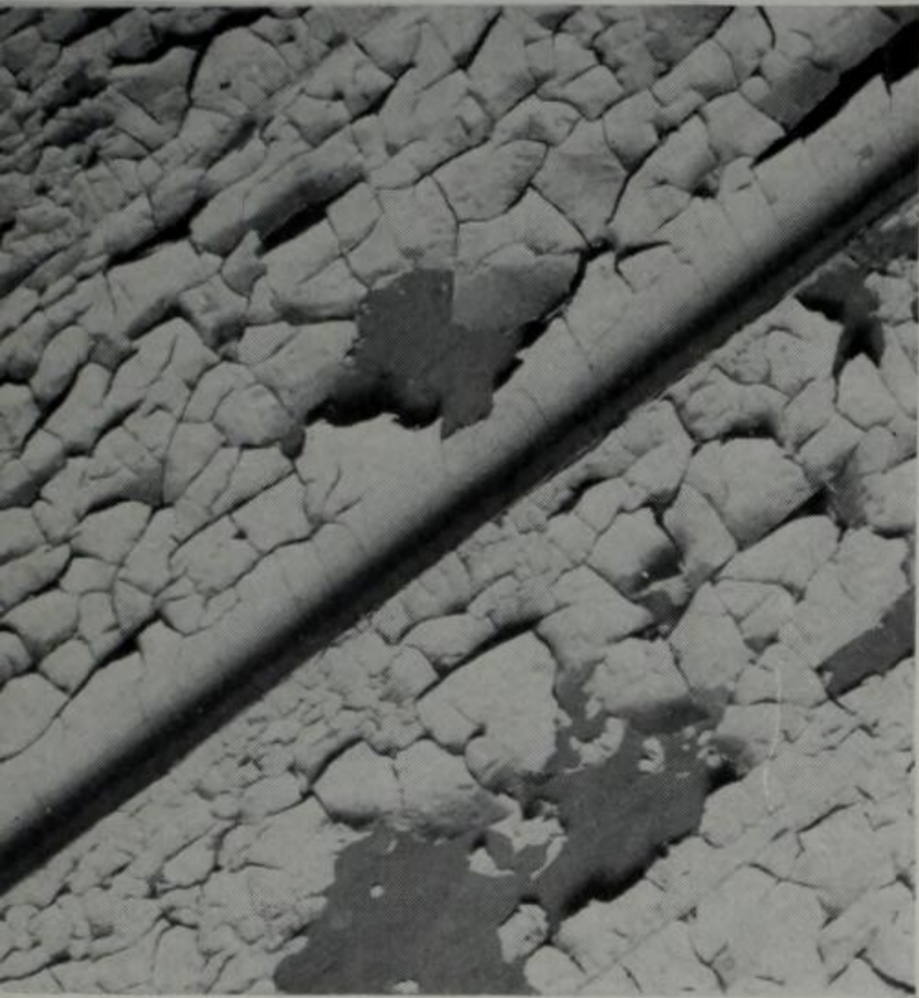
Fig. 3. O Harvey J. Croze, 1944 Peeling paint
