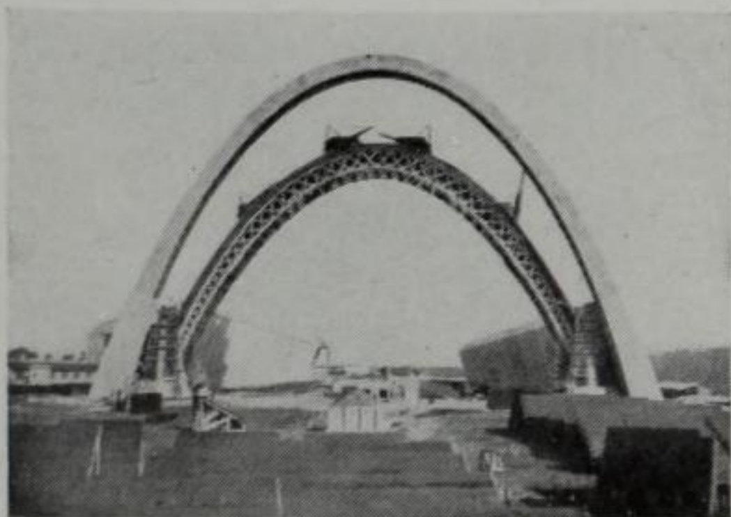
Fig. 133. Gustave Freyssinet, 1914 Reinforced concrete hangar for a dirigible in Orly, France The arches constructed under the direction of the engineer allow tremendous inside space without disturbing columns
