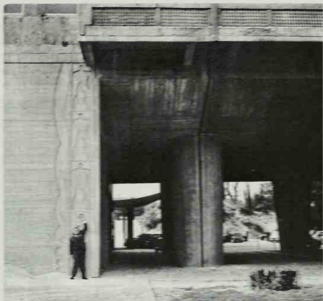
The colossal underpinning of Le Corbusier's Marseille block, four men high See also illustrations page 174
