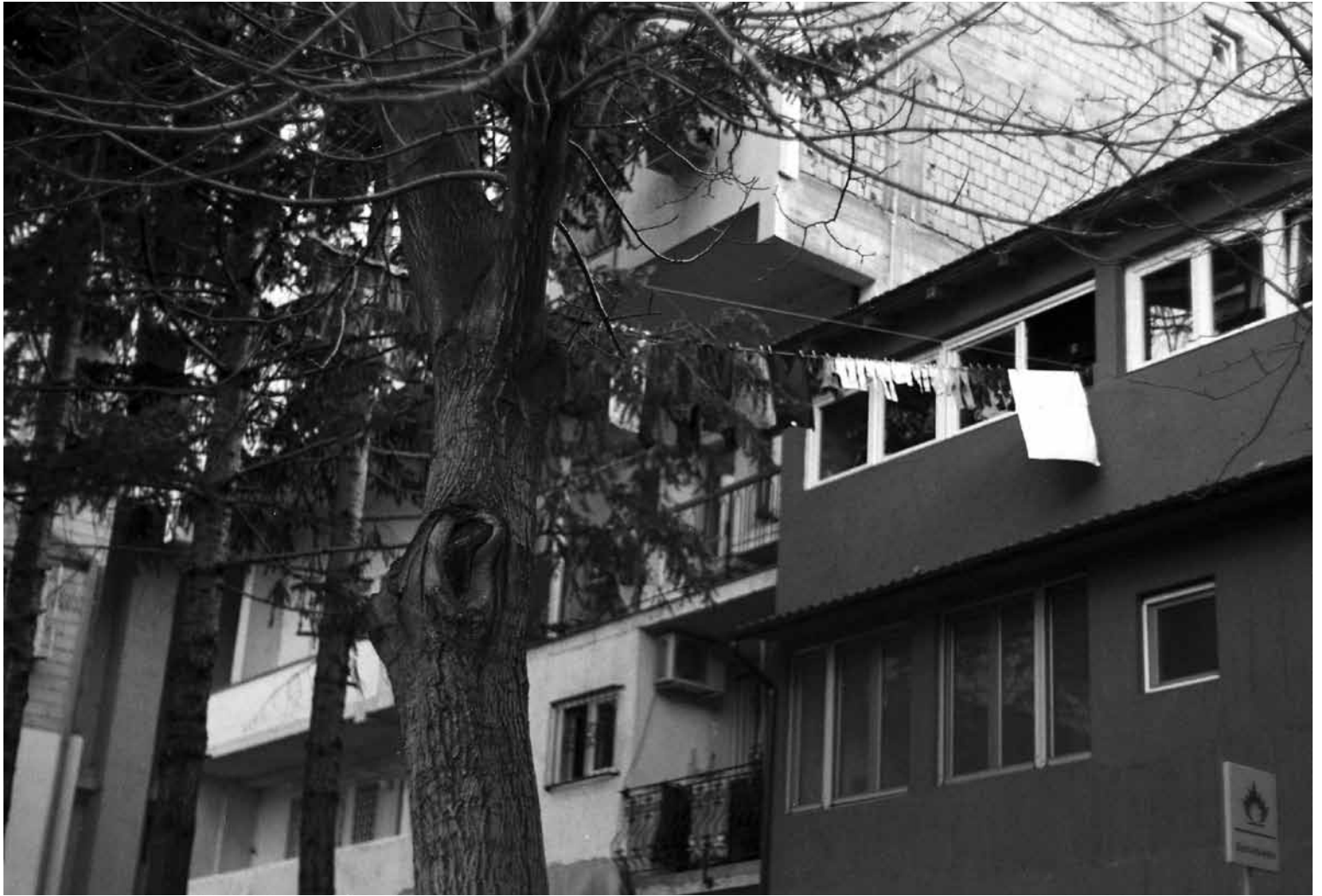
The side wall of this Russian Pavilion extension is left unfinished in anticipation of a neighbouring extension that was never built, leaving exposed brick without any insulation or facade finish.
