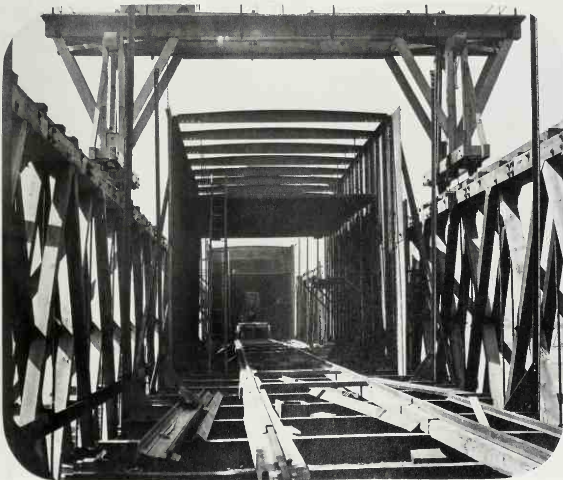
183. WILLIAM NOTMAN. Victoria Bridge, Framework of Tube and Staging, Looking in, May, 1859. Albumen print. Notman Photographic Archives, McCord Museum, McGill University, Montréal.
