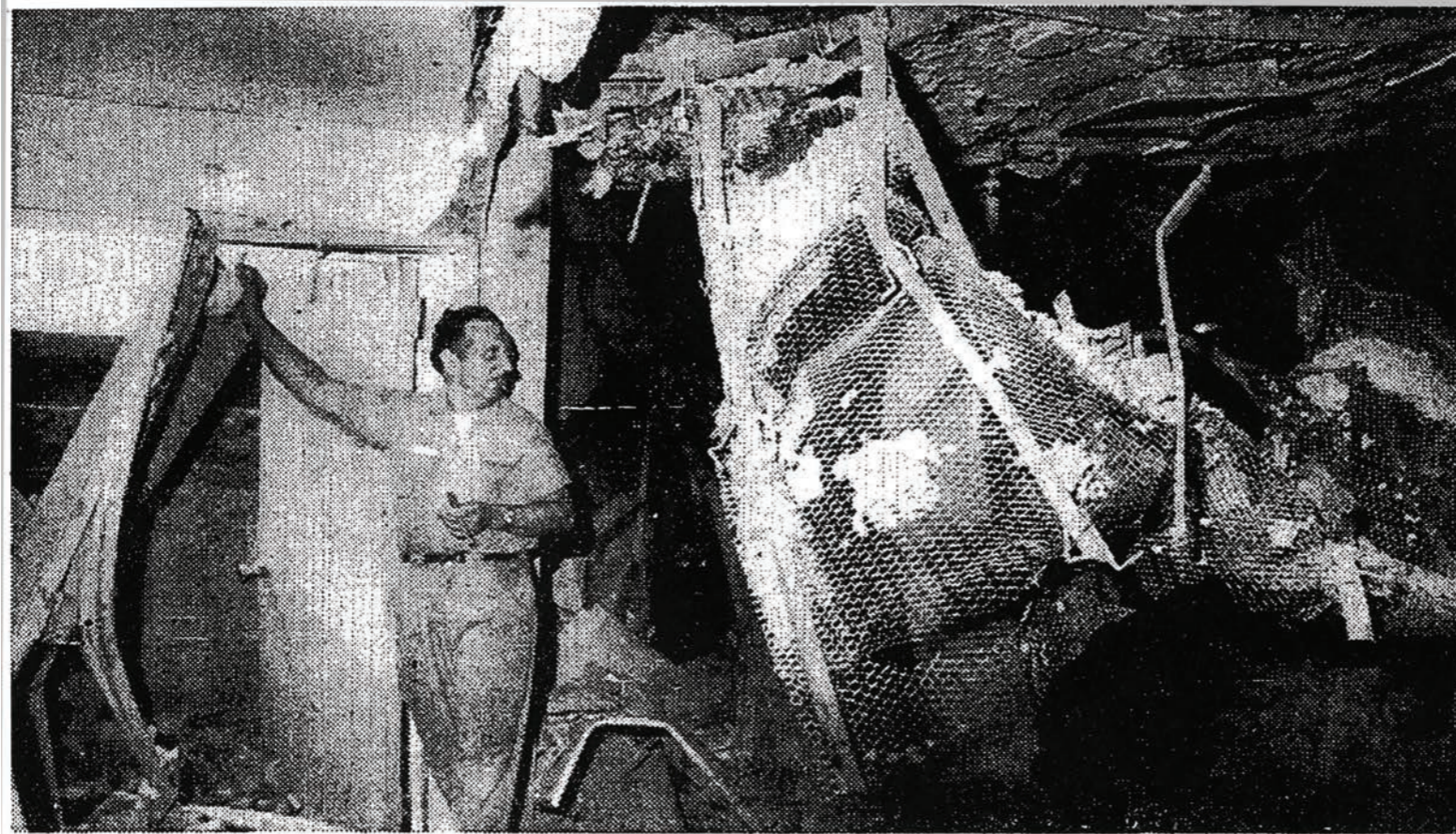
AT GENERAL TELEPHONE BUILDING: A plumber surveying damage on 21st floor before starting to make repairs
