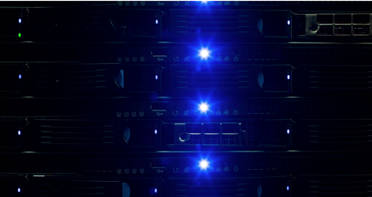
Data Center Observatory, Carnegie Mellon University. Photo © Jonathan Minard. Used with permission.
