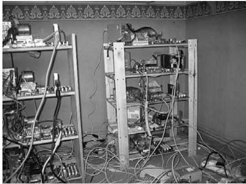
DIY datacentre, when the network becomes tangible again.
