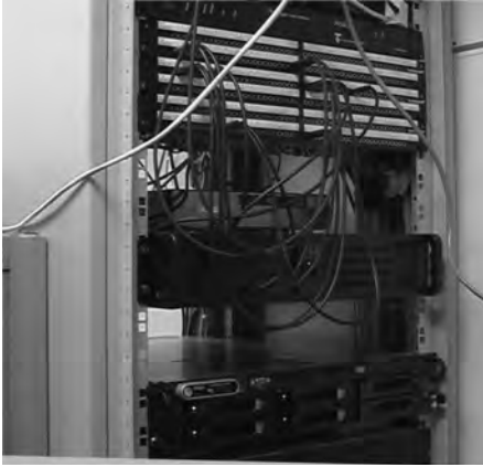
An analog studio—devices are connected with cables.
