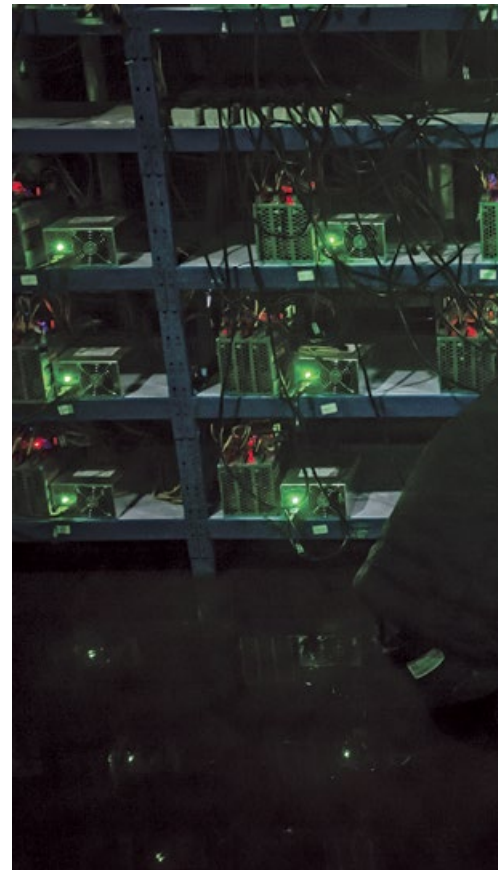
right: A worker inspects a malfunctioning mining machine during his night shift. Miners can check a machine's condition and operations using phones and personal computers. For most issues they can simply restart a machine.
