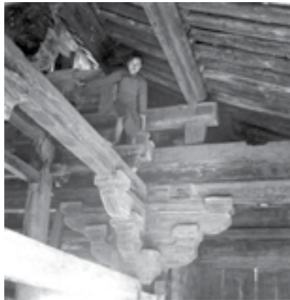
Lin on the beam of the Bell Tower of Kaiyuan Temple, Zhengding, Hebei, 1933
