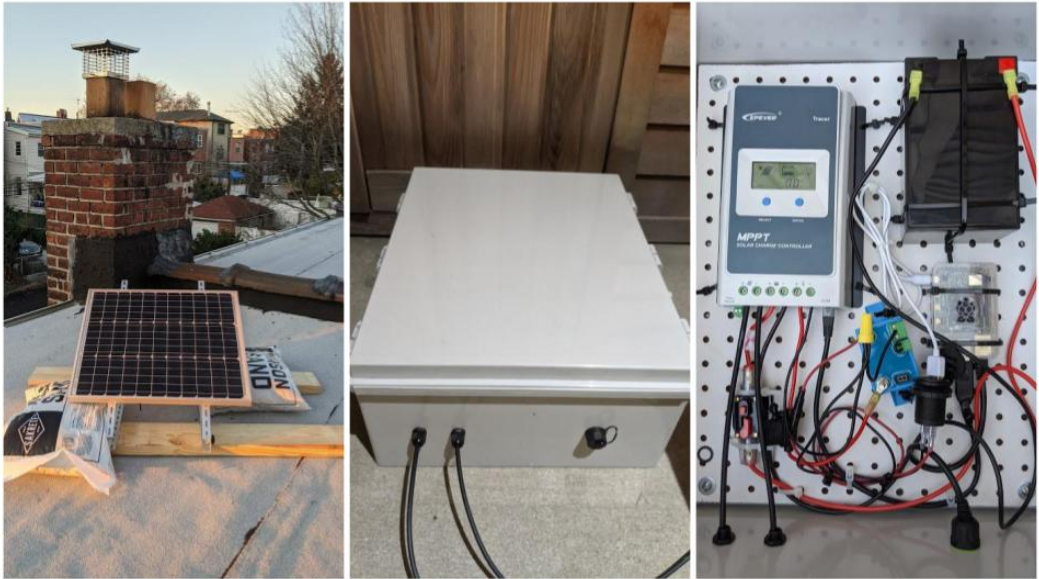
Fig. 2. A solar-powered server installed on the roof of a building and its components
