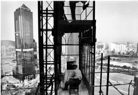
Liang Juhui. One Hour Game . November 1996. Color photograph of performance at skyscraper construction site, Tianhe, Guangzhou
