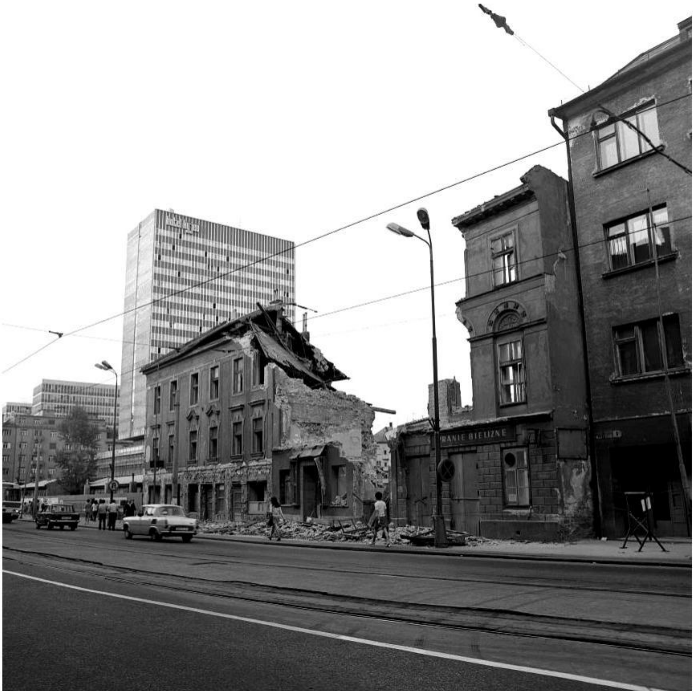
Demolition of the original structure on Špitálska ulica after the completion of II. stage of construction of the commercial-social centre, 1973 Source: Department of Architecture archive, Institute of History, SAS
