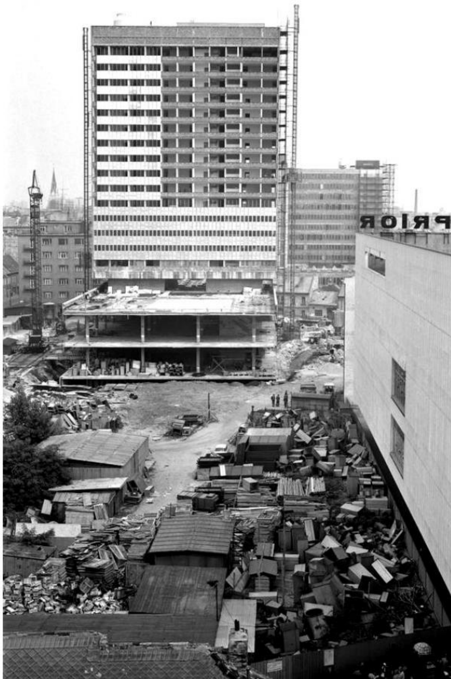
Construction of Hotel Kiev, around 1971 Source: Department of Architecture archive, Institute of History, SAS
