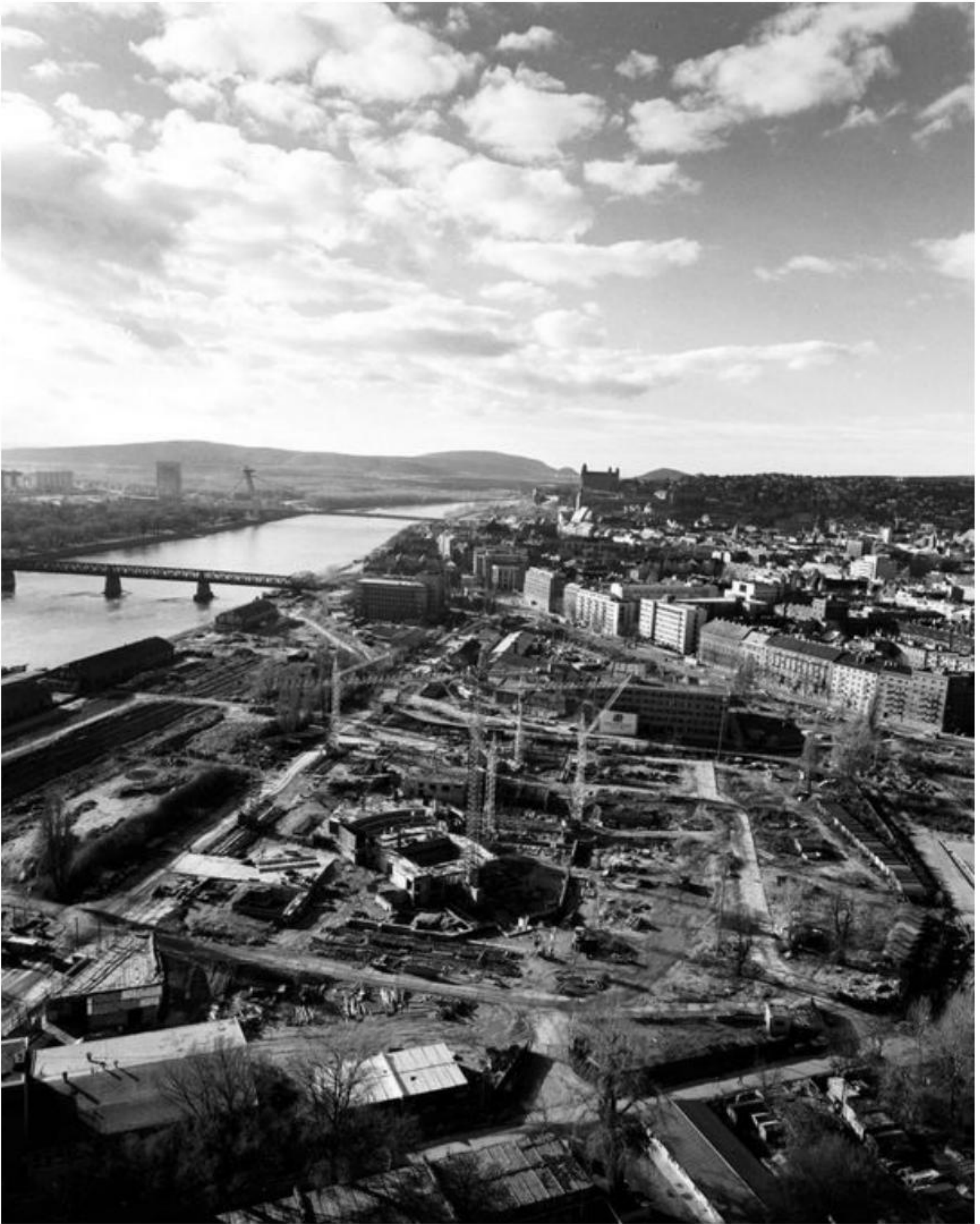
Construction of the Slovak National Theater, around 1988 Source: Department of Architecture archive, Institute of History, SAS
