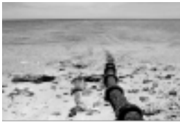
Tumon Bay Cable Landing Station
